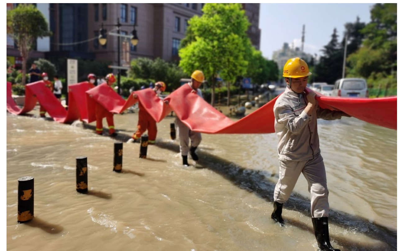
▼ Pioneer Commando consisting of the Party members in China United Cement Dengfeng Co., Ltd participated in the laying of drainage pipeline at the rescue point.
